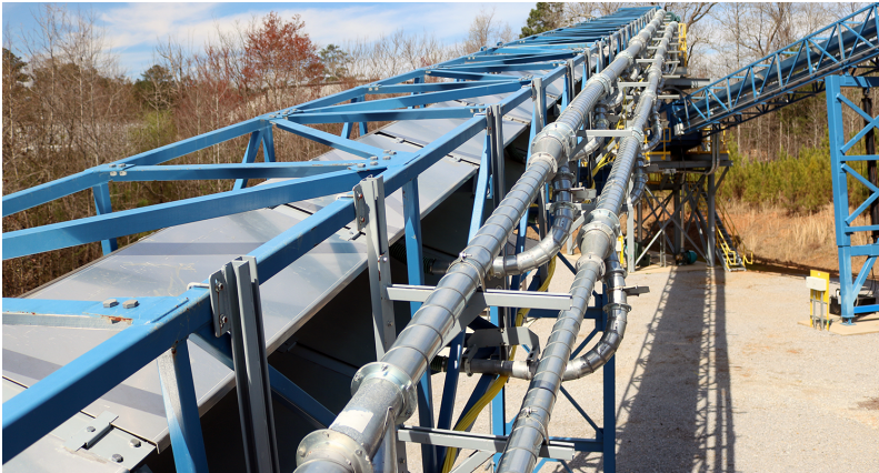
AIR SUPPORTED BELT CONVEYORS
