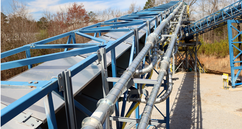
AIR SUPPORTED BELT CONVEYORS
