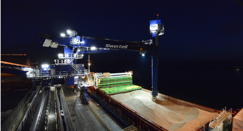
SHIP UNLOADER - DENMARK
