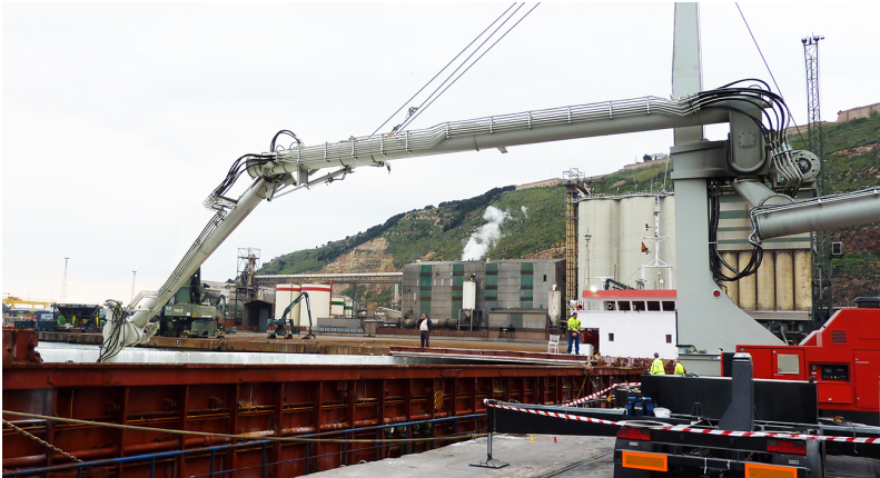
MOBILE UNLOADER - SPAIN
